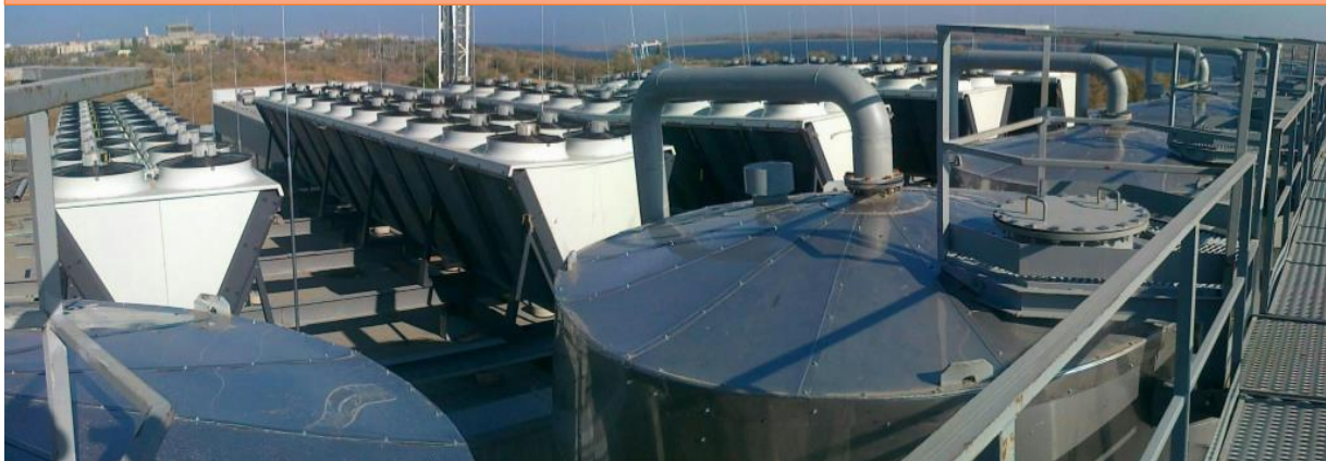
Shopping center Aquarelle, Volgograd Energy center using cold accumulators
